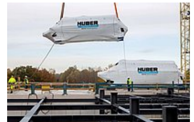
After the dryers have been lifted into place, the steel construction above the dryers can now continue
