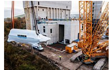
The dryers are lifted directly into the building onto the prepared level
