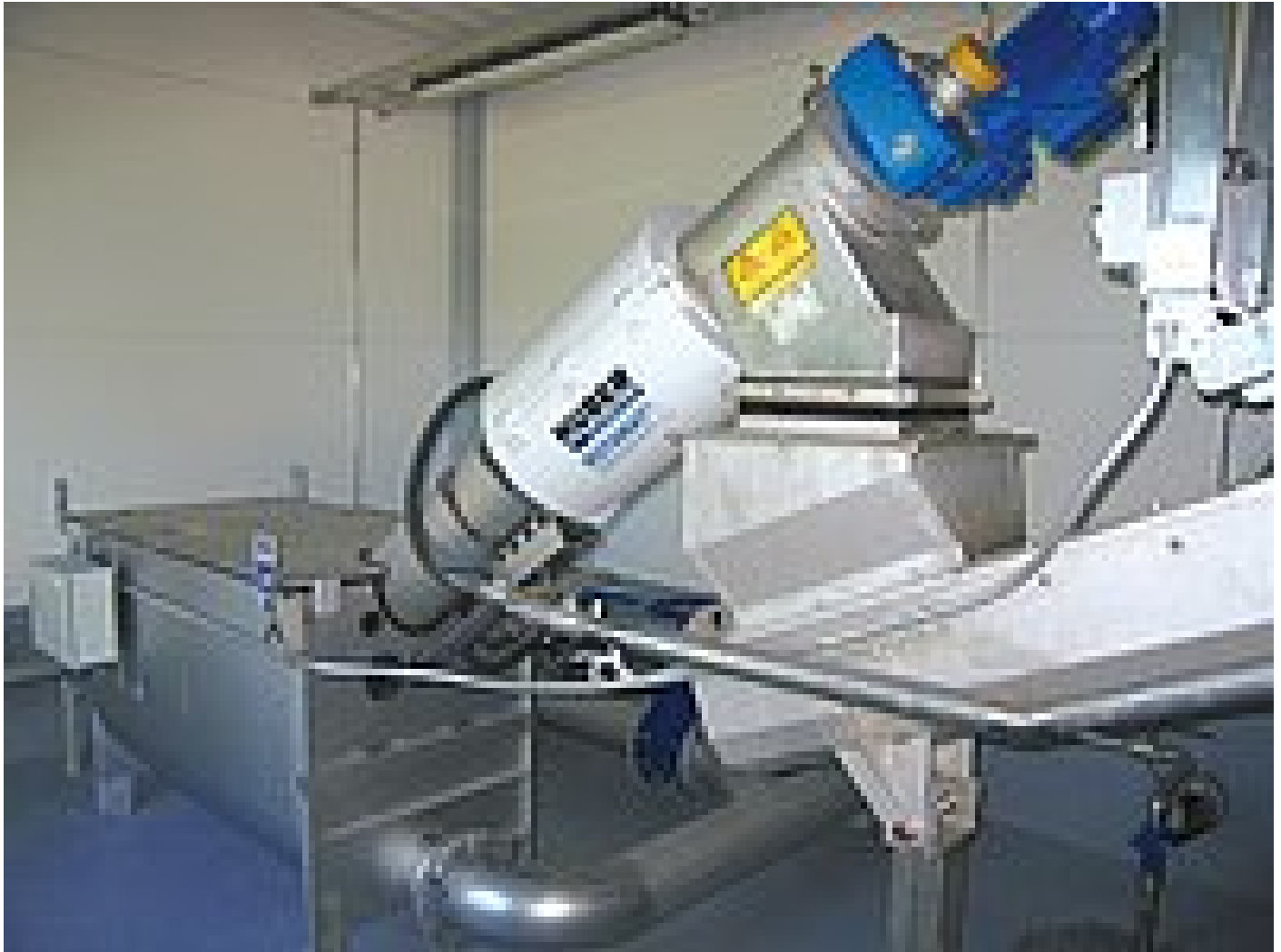
Septage receiving station Ro 3 with integrated IRGA for screenings washing and enclosed Ro 8t screw conveyor forwarding the screenings to wash-press WAP/SL
