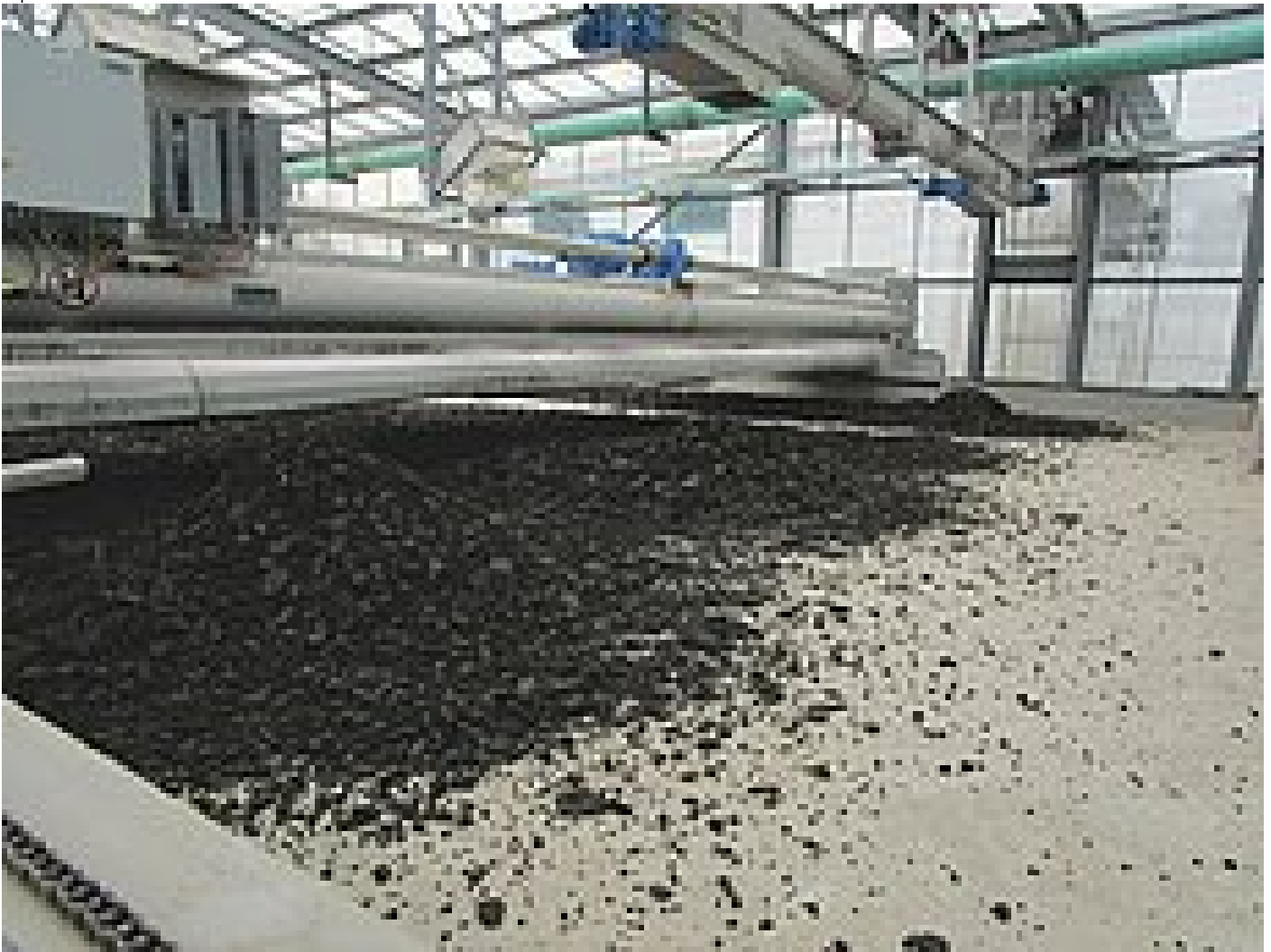
The new SOLSTICE® 11 turning sludge at Zhenjiang, China
