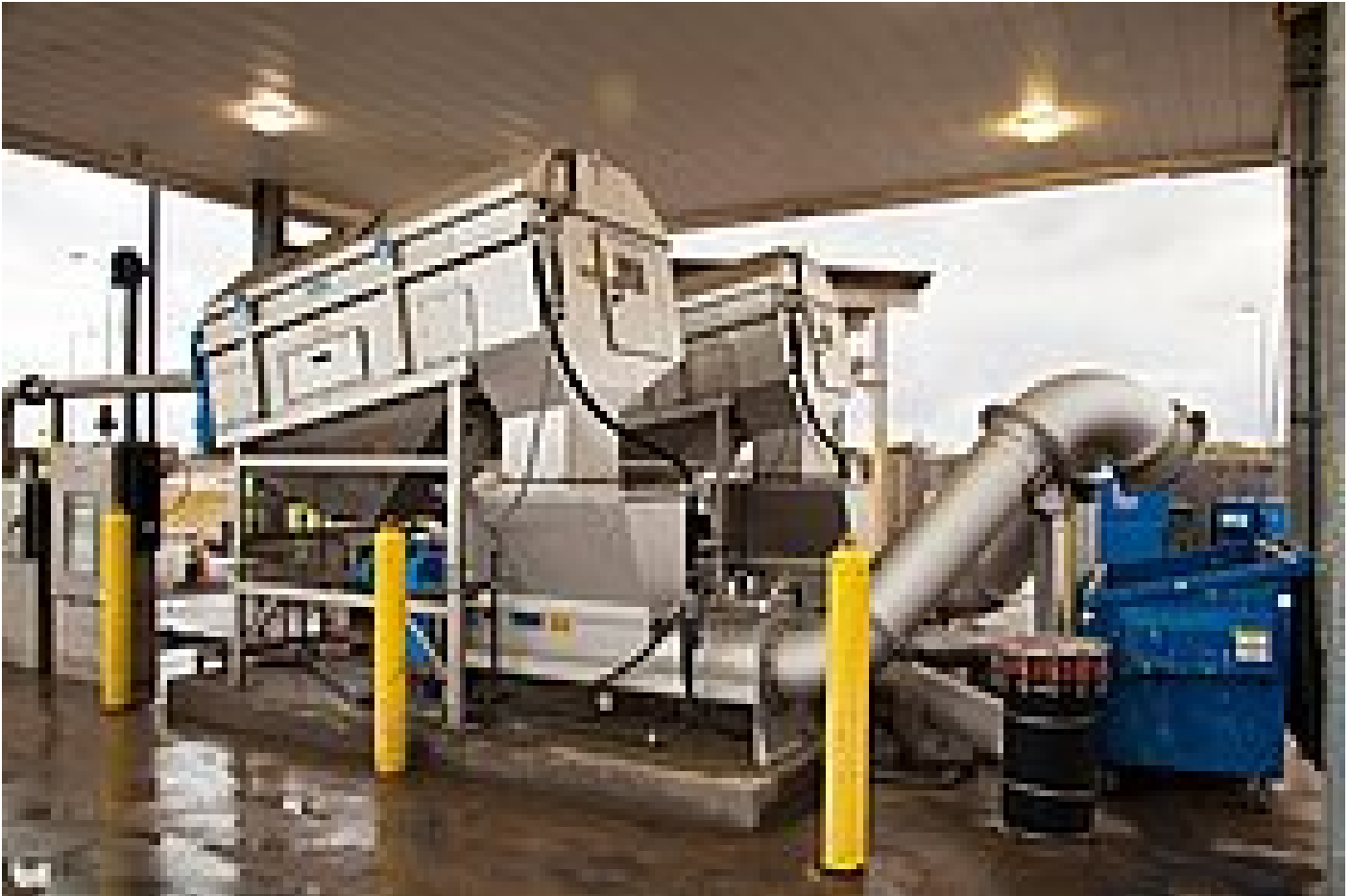
HUBER Sludge Treatment products in the San Antonio receiving station process
