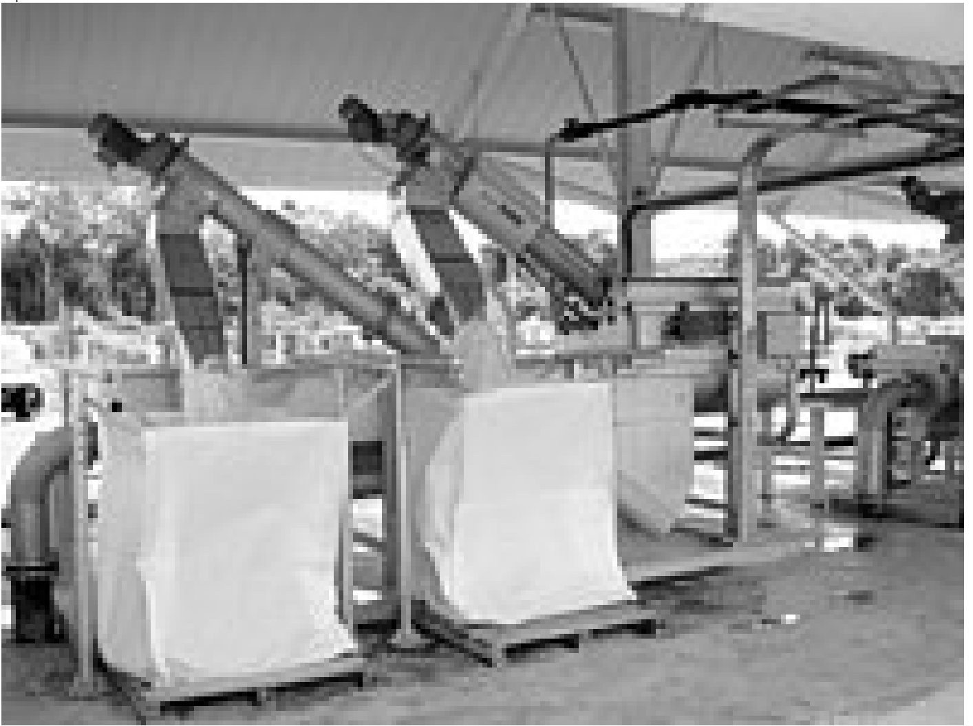
Complete mechanical preliminary treatment: removal of screenings and grit by the HUBER ROTAMAT® plant
