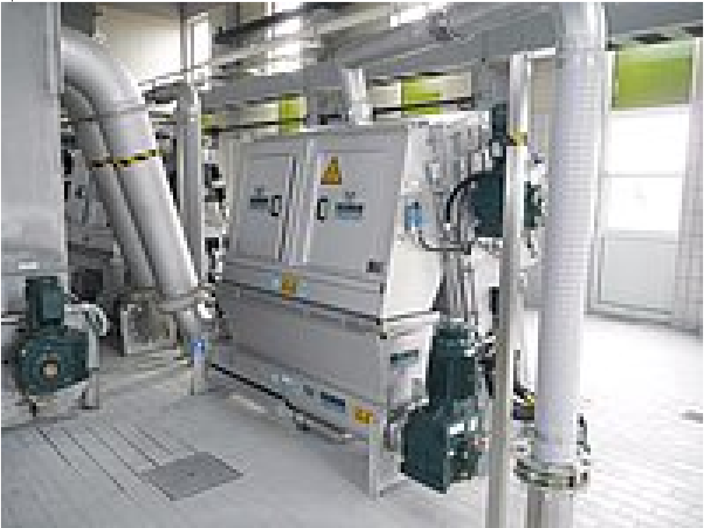
Discharge end of the coarse screen with wash press
