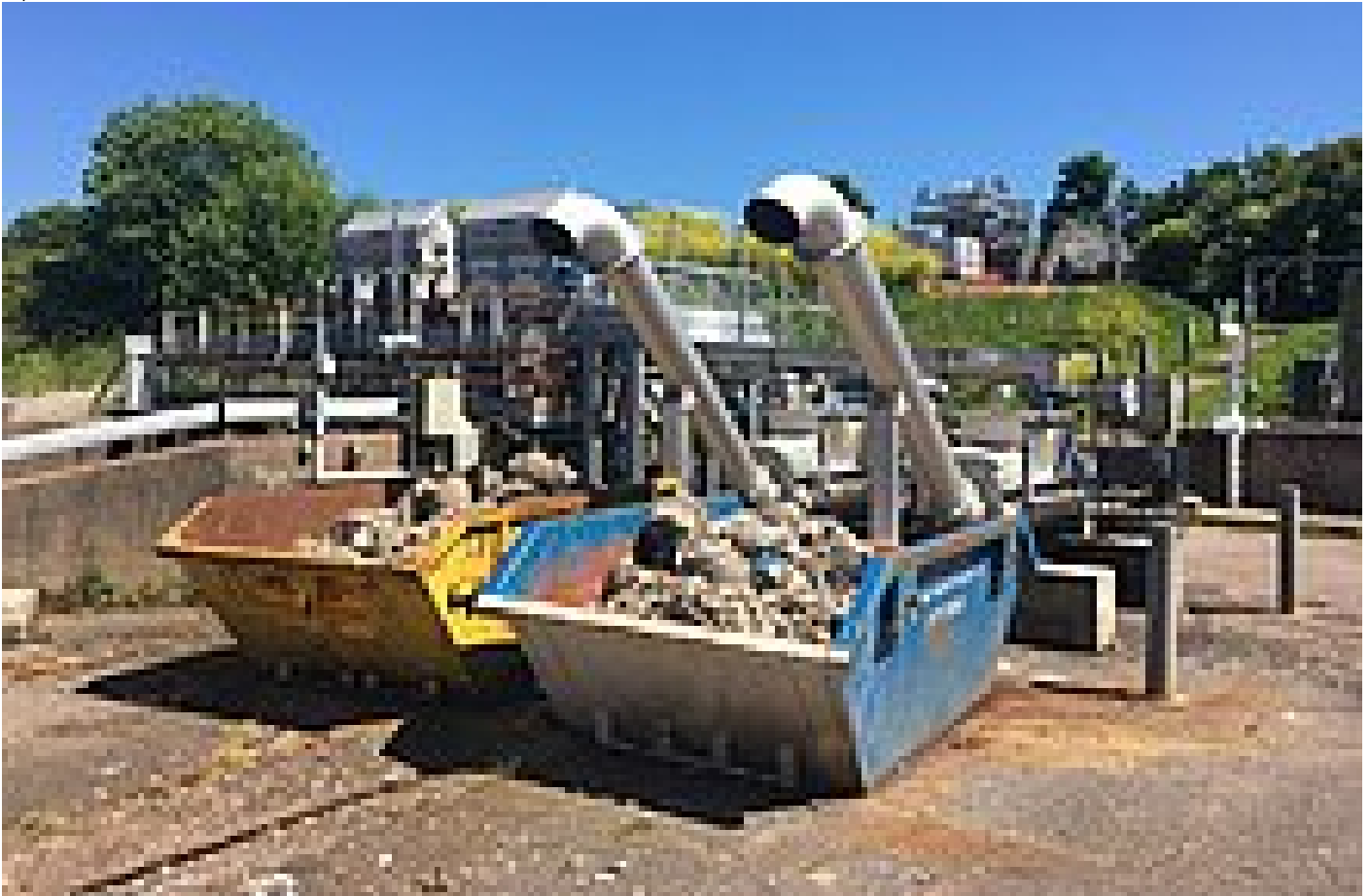
New HUBER Wash Press WAP®-L BG4v screenings handling plant, EscaMax® inlet screens and RakeMax® bar screen in the background
