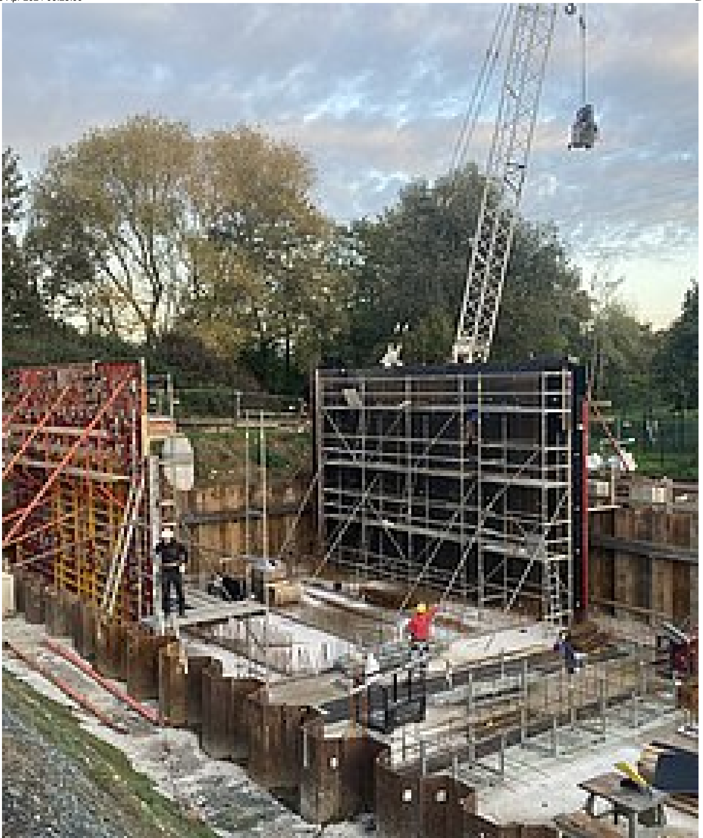
Construction of the activated carbon filter stage in Bickenbach is progressing. (Photo: Jörg Stanzel, Wastewater Association Bickenbach)
