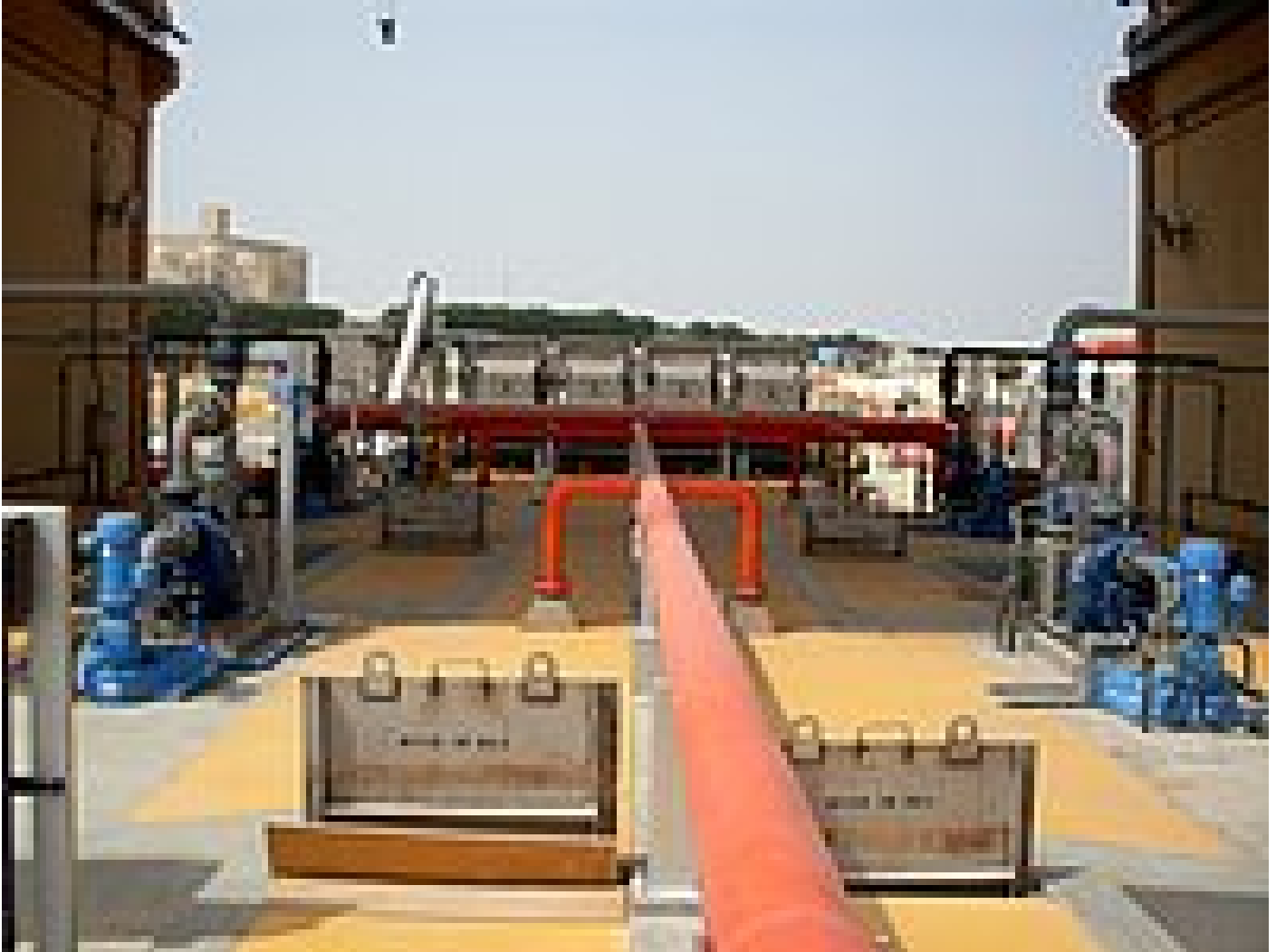
Installation with a set of 4 VORMAX units
