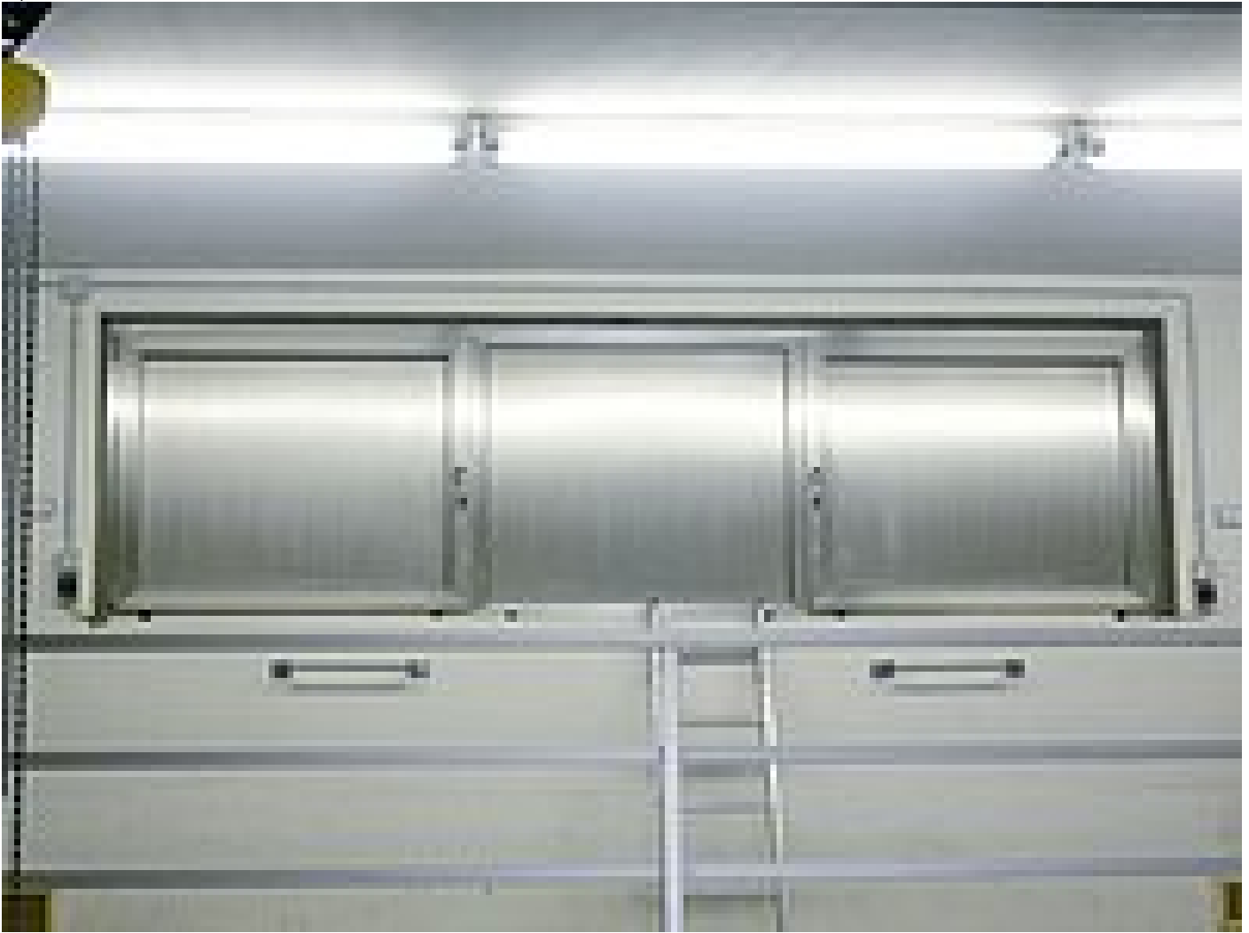
Stainless steel window in elevated reservoir
