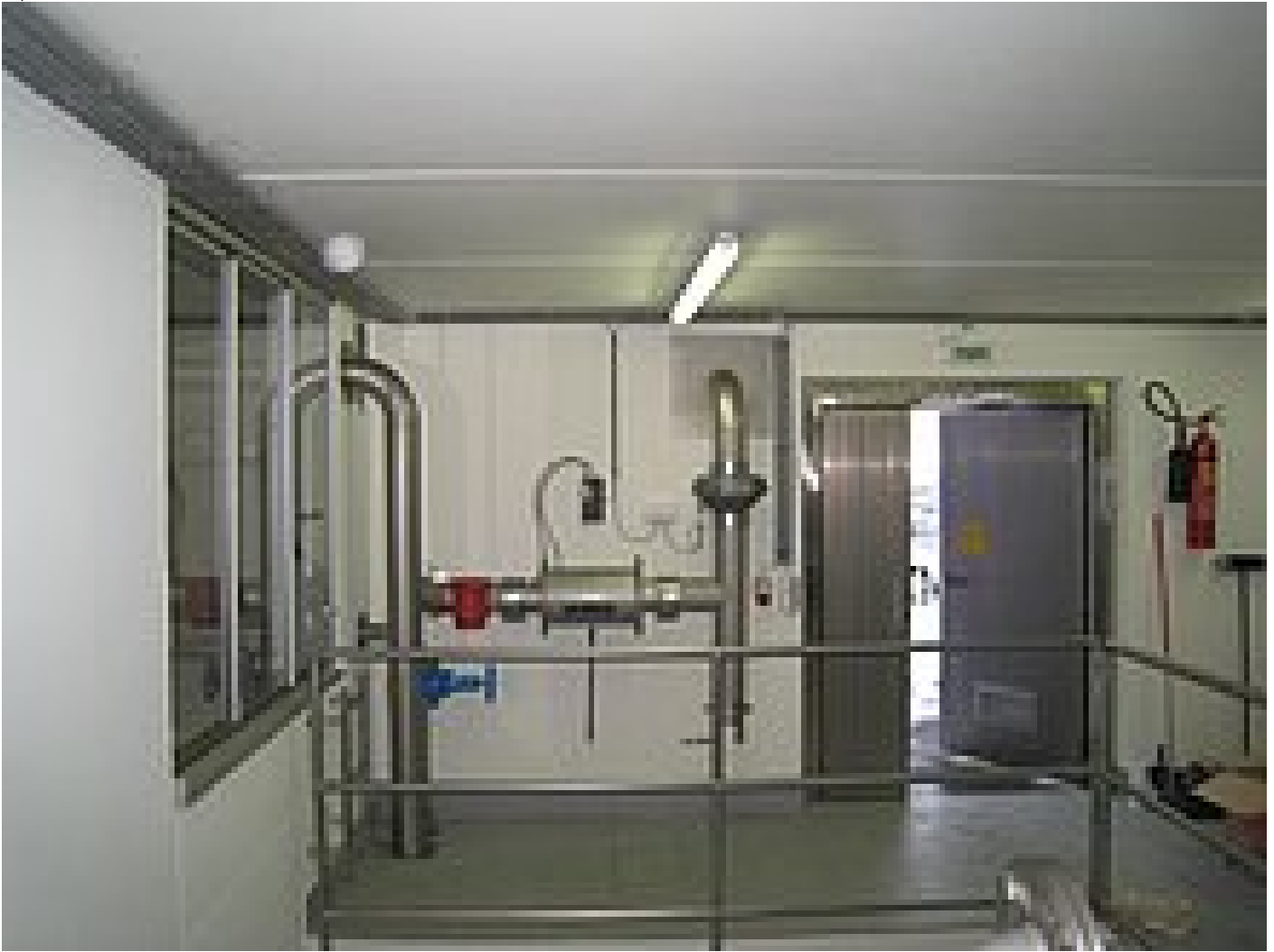
Utzenaich – in flow direction: wall connection plate in the safety louvre (outside not shown), air suction line to the radial pipe ventilator with 5-stage transformer for rotary speed variation, L251 air filter plant (with differential pressure switch), safety valve type 170-1 (red, approx. 1,000 Pa triggering pressure)
